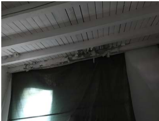
Figure 6: Moisture damage on the ceiling of the Sepulveda Room
