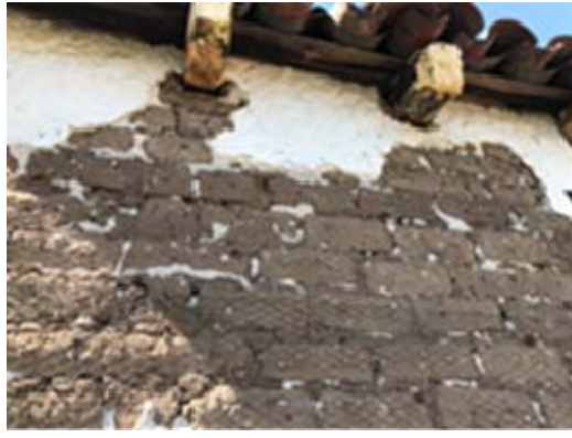
Figure 2: Delaminated plaster, exposed adobe bricks and deteriorated rafter tails
