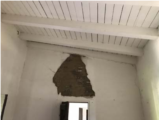
Figure 3: Delaminated interior plaster and exposed adobe bricks
