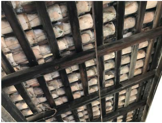
Figure 7: Damaged clay roof tiles in the Corredor with no underlayment or sheathing
