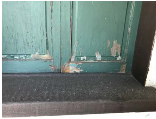
Figure 8: Deteriorated wood door in need of rehabilitation
