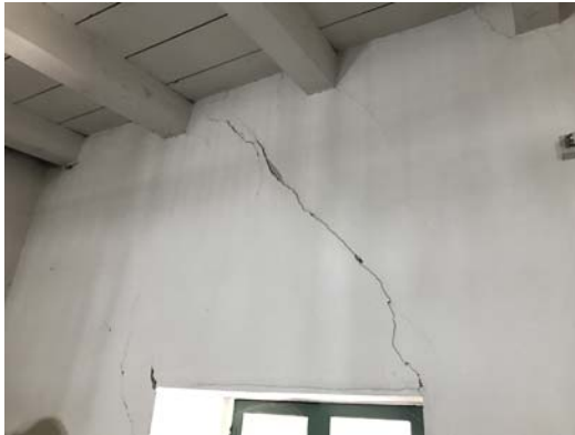
Figure 4: Interior wall crack
