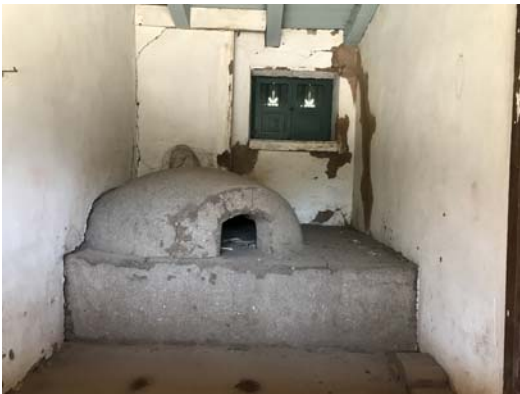
Figure 5: Interior cracks and moisture damage in the Horno
